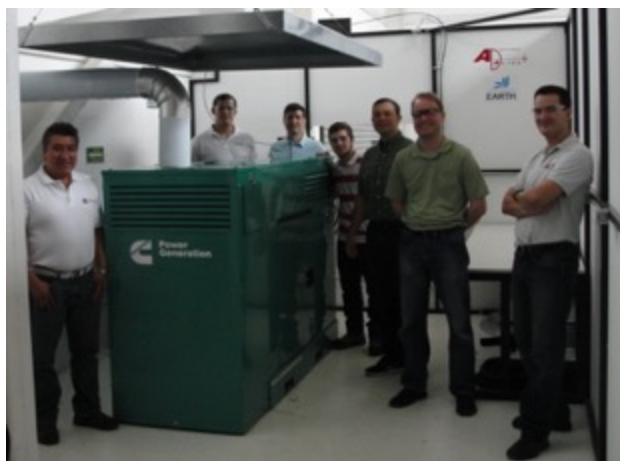
Ad Astra – Cummins hydrogen biogas power generator. Source: Ad Astra Rocket Company
