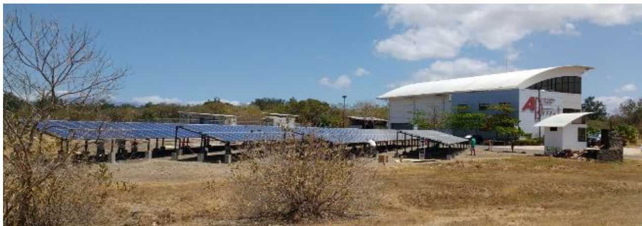
Ad Astra, Costa Rica completed a 76-kW solar installation designed to supply 100% of its electrical power needs. Source: Ad Astra Rocket Company
